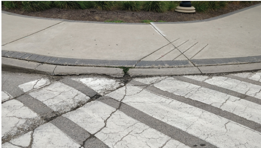
The curb cut at Stearn Drive and Michell Crescent is difficult for those with mobility devices to navigate across due to large cracks and uneven paving.
