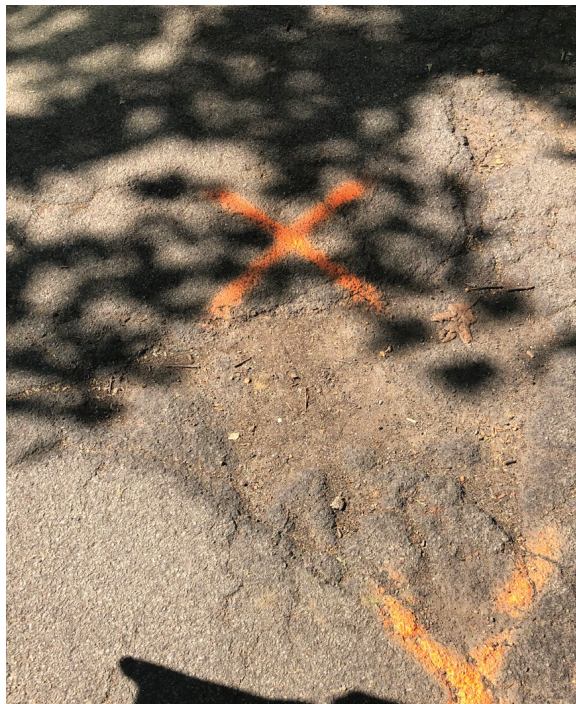
One participant photographed areas where tripping hazards have been indicated with spray paint, but not repaired.
